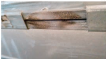
Condensate leak at flange
