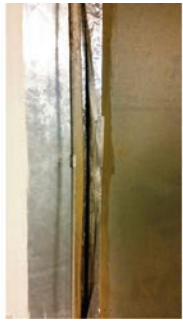
Duct tape blown away
