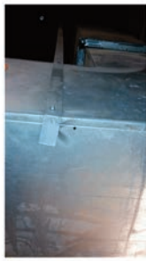
Unsealed holes at hangers
